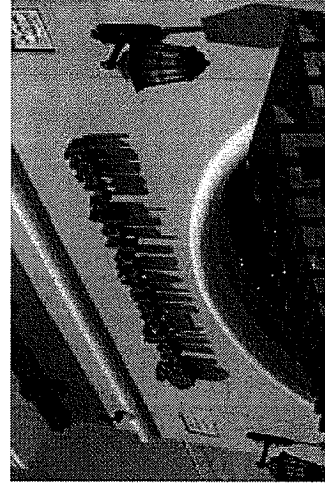
Signage with LED lighting.
